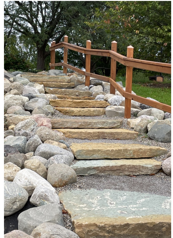
Our Educational Gardens underwent major renovations in 2024, new raised bed gardens, an additional walking trail and steps were added connecting existing walkways to trail around the lake. The gazebo was replaced using the top of a reclaimed grain silo from a farm in Utica, KY and a prairie buffer was planted around the lake.
