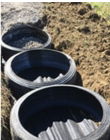
Figure 4. Nonwoven geotextile fabric and tread cylinders are placed in a trench and backfilled with dense-grade aggregate (DGA).
